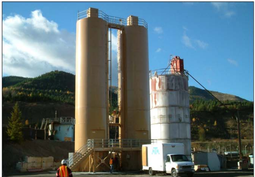
ZMI/Portec's new water treatment system installed at the Bunker Hill job site in Kellogg, Idaho.
